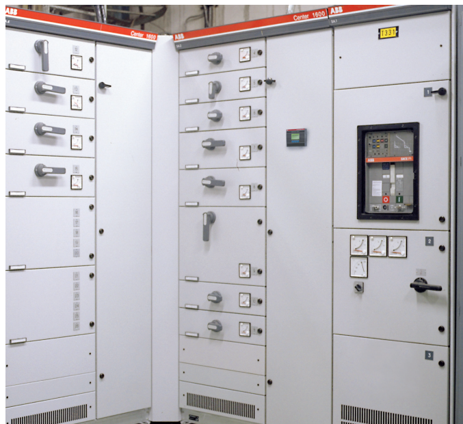
Arc Guard System™ – TVOC-2 installed in an ABB Low Voltage Switchgear
